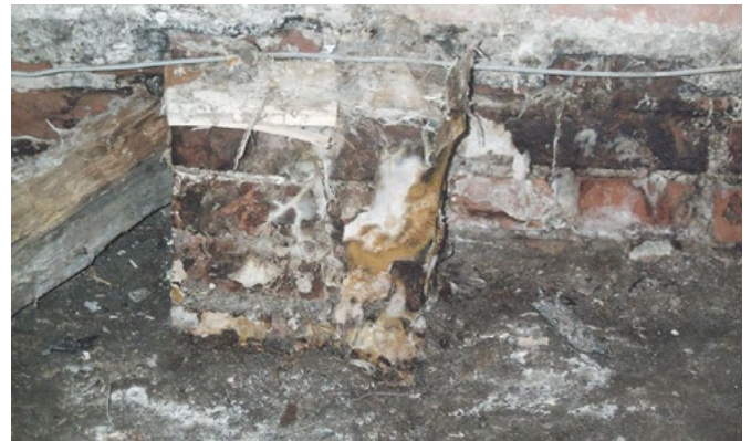
Development of mold and damage to the fabric of the structure
